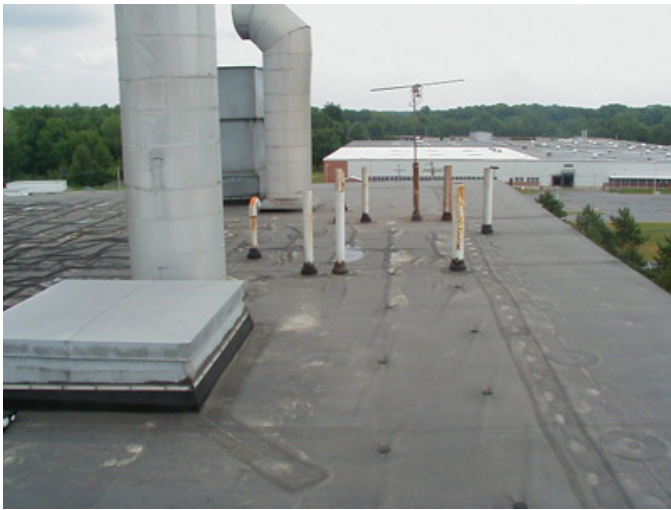
Old mechanically-attached EPDM roof system
